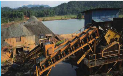
The crushing plant
